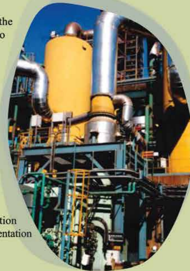
Dynamic pressure measurements in a centrifugal blower in steel work to analyze the reasons for several impeller damages
